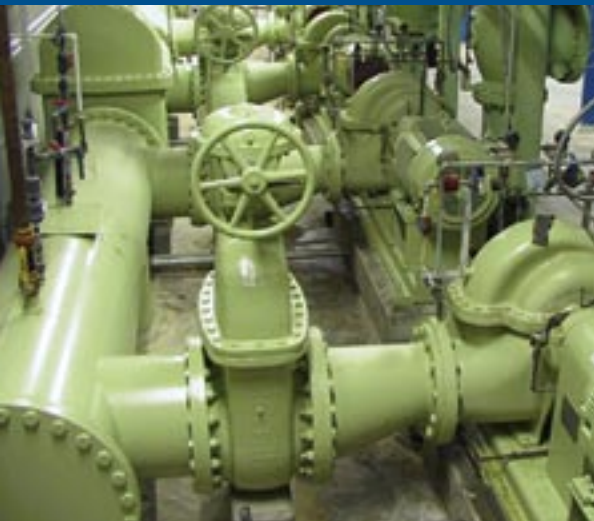
Water Pumps at Keokuk Municipal Water Works
