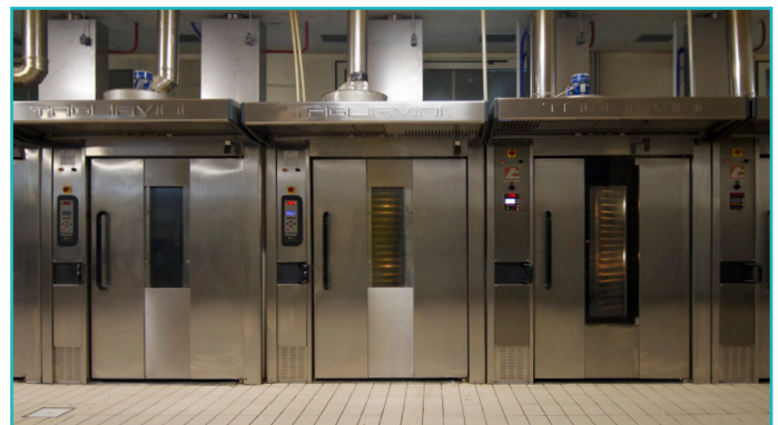
Ovens at Drago's Facility
