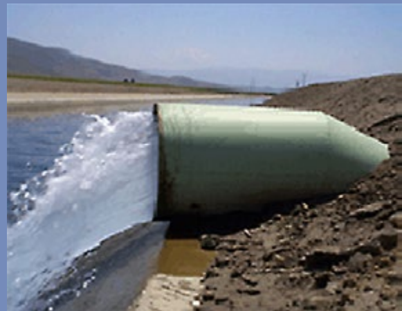
Water Transfer from Ground Storage
