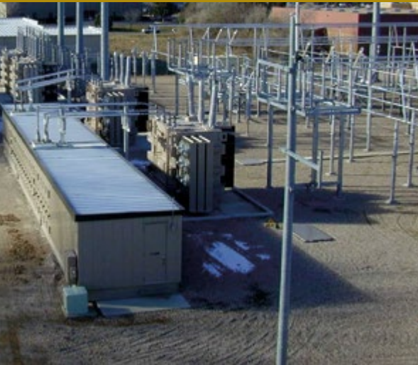
A Fort Collins Utilities Monitored Substation
