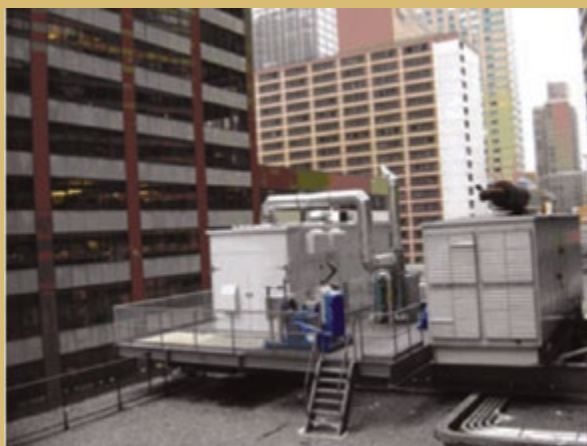
A DFC300 Installation in Downtown Manhattan
