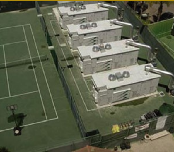
Fuel Cell Energy DFC 300s on a San Diego, CA tennis court
